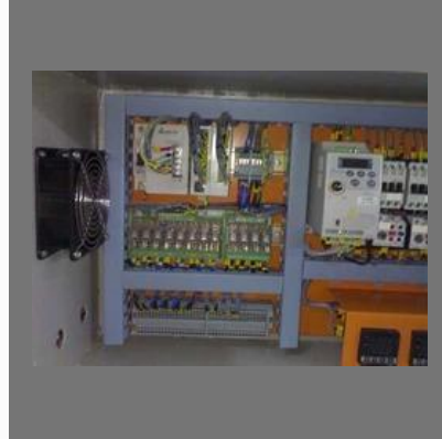
Automation Control Panel
