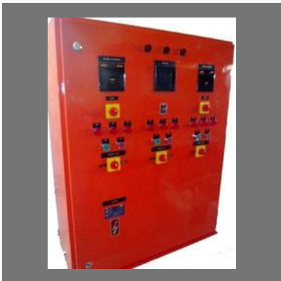
Fire Fighting System Control Panel
