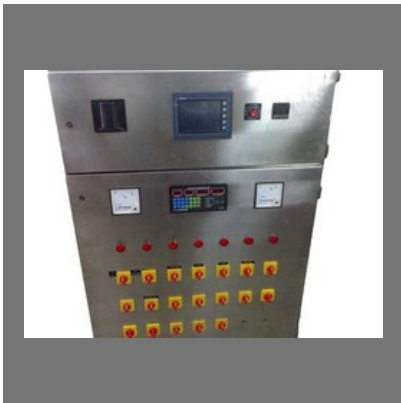
PLC Yarns Dyeing Panel
