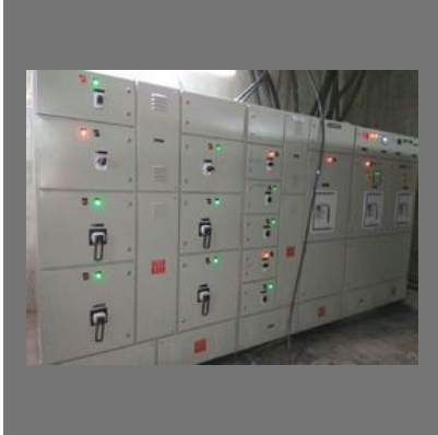
PCC Control Panel DB Panel
