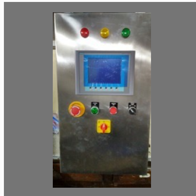
Liquid Plant Panel
