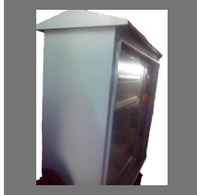
Distribution Control Panel
