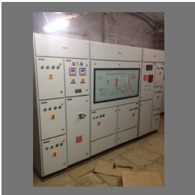
Power Control Panel APFC
