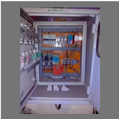
Sab Pump Electrical Panel
