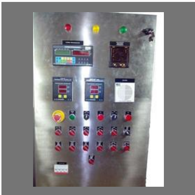
Yarn Dyeing Control Panel
