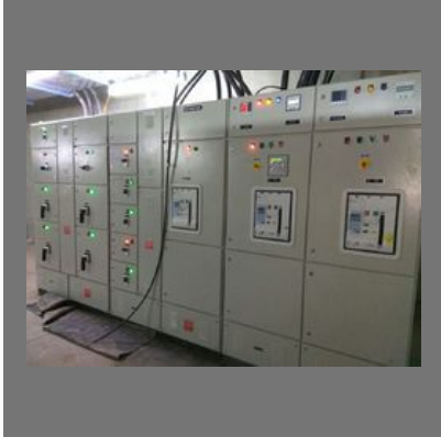
PCC Control Panel DB Panel
