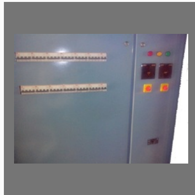
Outdoor Electrical Panel
