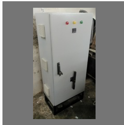
50HP Compressor Control Panel with VFD
