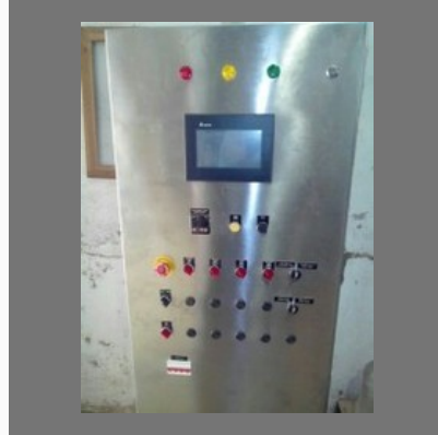
PLC Yarn Dyeing Control Panel
