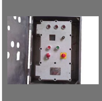
FLP Vaccume Control Panel
