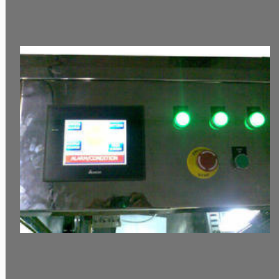
PLC Tablet Punching Control Panel
