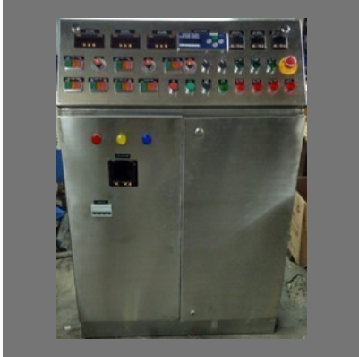
Oilment Plant Control Panel
