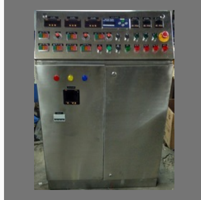
Ointment Plant Control Panel
