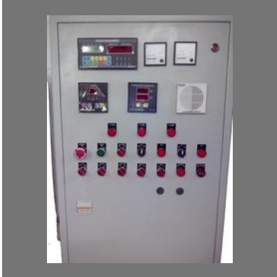
Electric Control Panel
