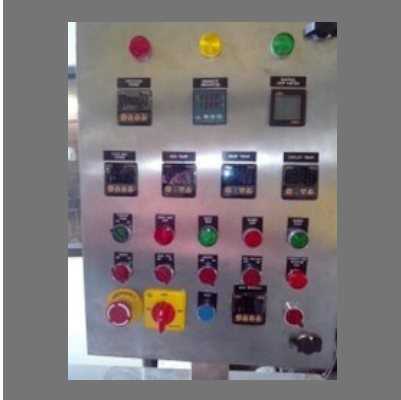
FBD Control Panel
