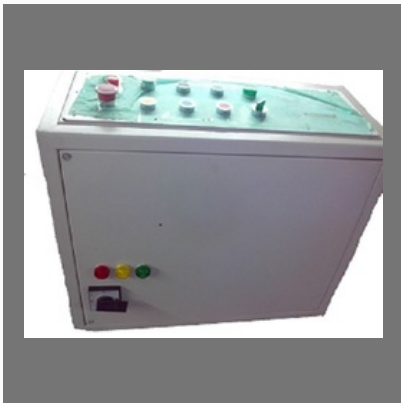
Shrink Tunnel Control Panel
