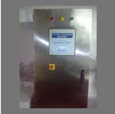
PLC Soft Flow Dyeing Control Panel
